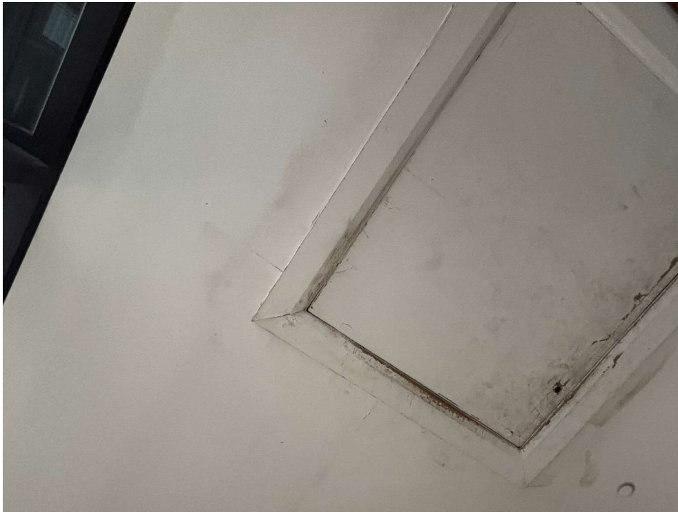
Photograph 3 - Typical Photograph of Water Ingress
