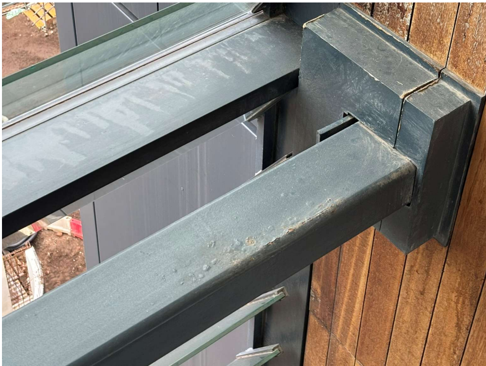
Photograph 2 - Typical Photograph of Surface Corrosion to Gridline C
