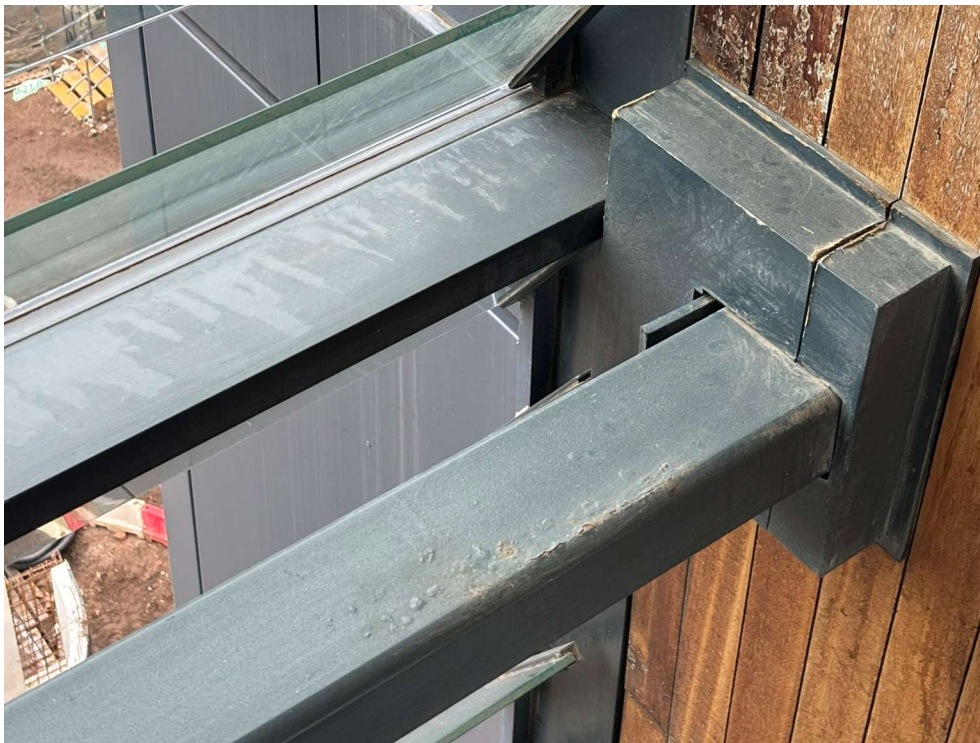
Figure 20 - Typical photograph of surface corrosion with corridors
