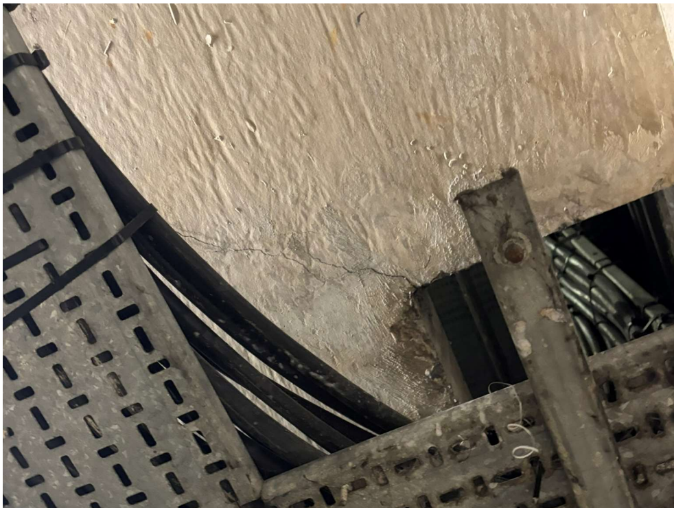
Photograph 16 - Hairline Shrinkage Cracking To Soffit Of In-Situ Reinforced Concrete Basement Floor Plate
