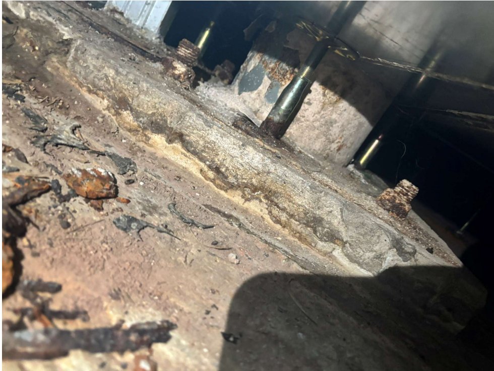
Figure 23 - Photograph of corrosion to baseplate just off Gridline 13H
