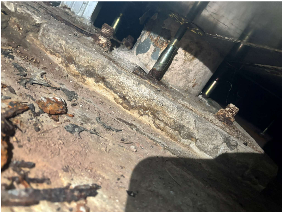
Photograph 8 - Corrosion To Column Base Plate
