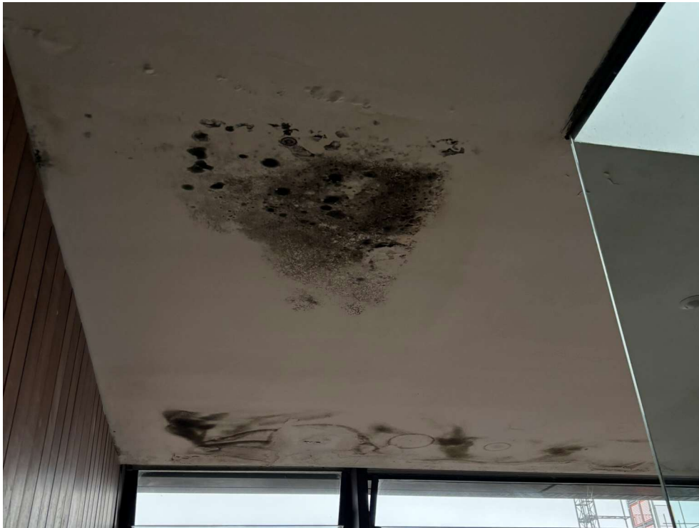
Figure 21 - Typical photograph showing evidence of water ingress, mould to soffit of roof construction
