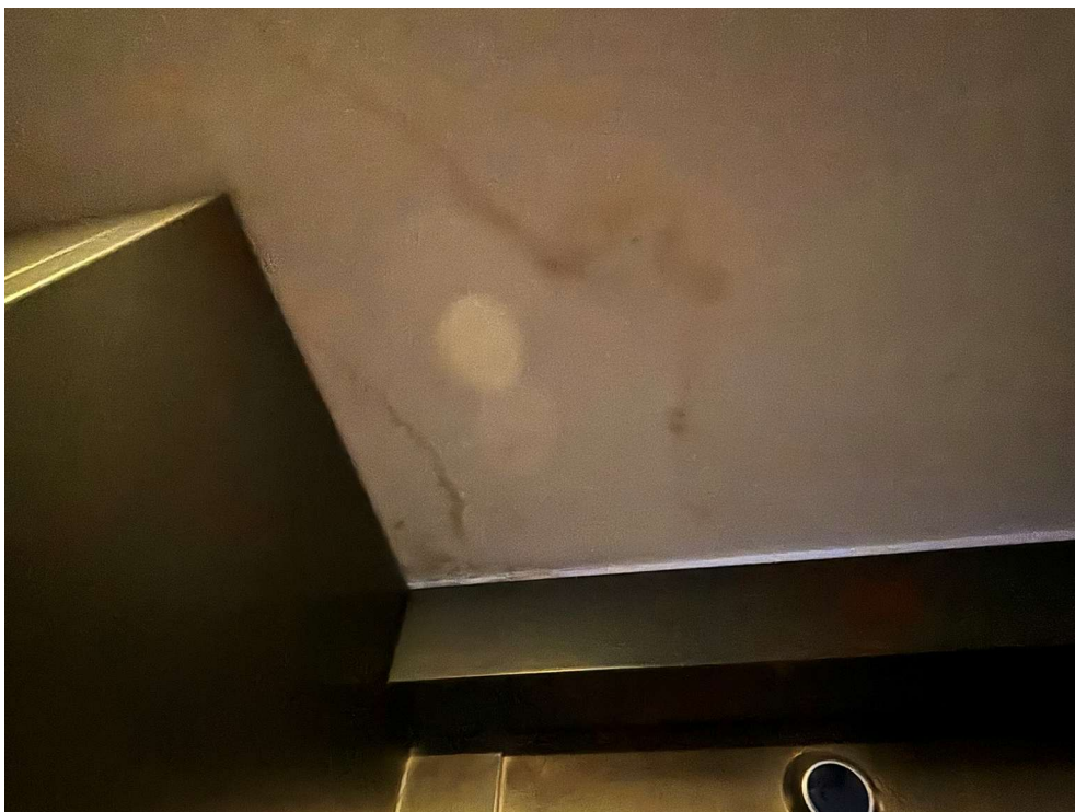
Photograph 4 - Typical Photograph of Water Ingress
