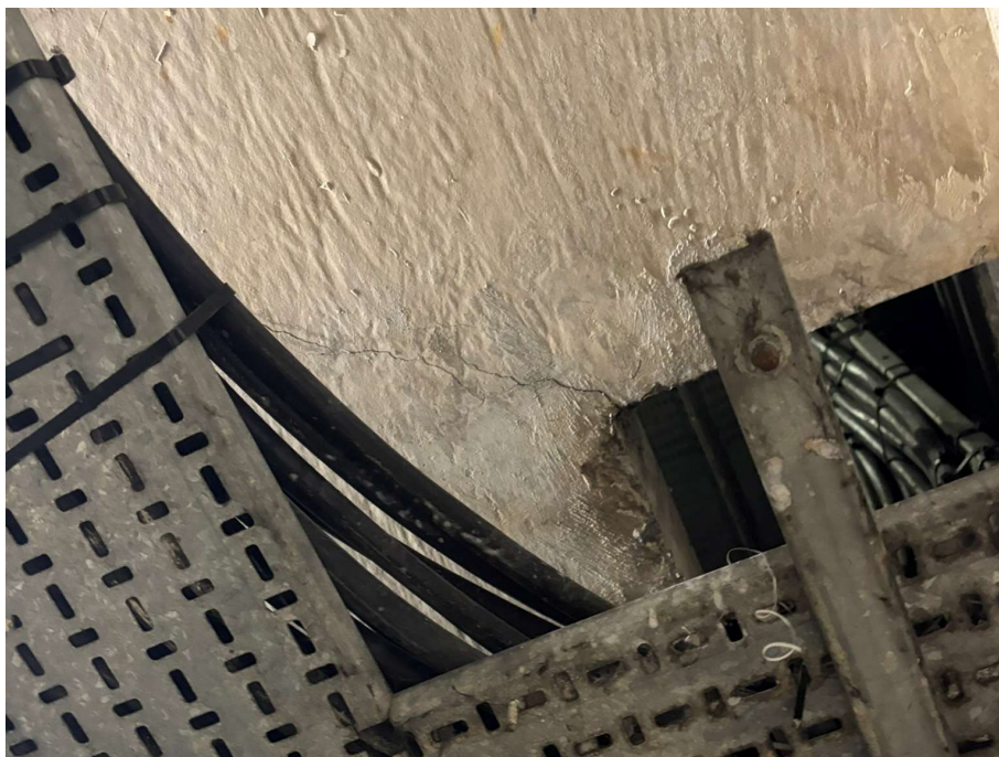
Figure 31 - Typical photograph of cracking to concrete basement slab at service penetration corner
