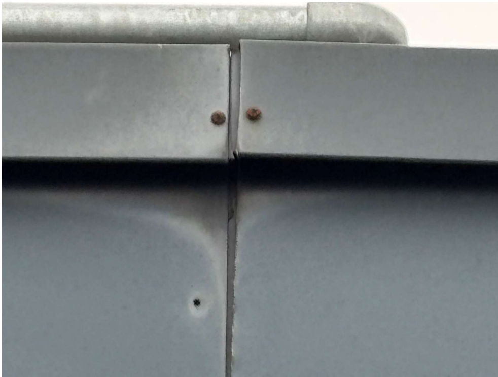
Photograph 19 - Missing Fixings To Cladding At Roof Level Gridline D
