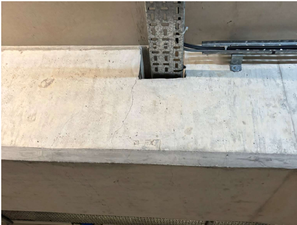
Photograph 15 - Hairline Cracking To Basement Concrete Beams Local To Service Penetrations
