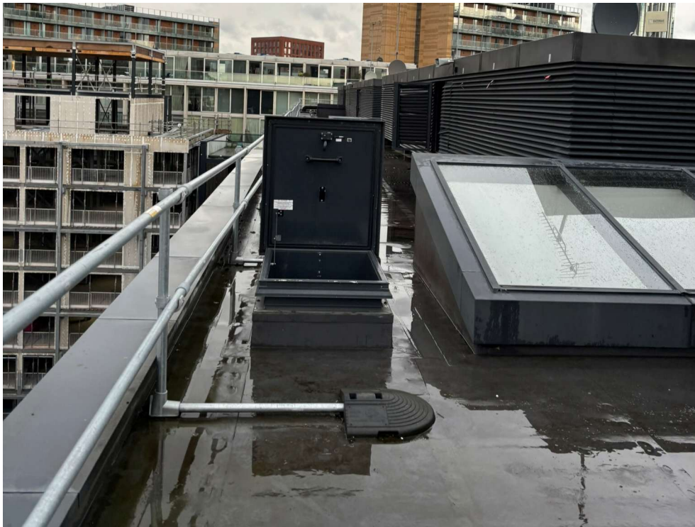
Photograph 11 - Ponding Water At Roof Level
