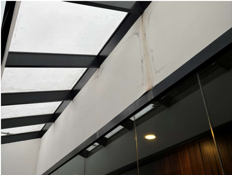
Photograph 5 - Typical Photograph of Water Ingress
