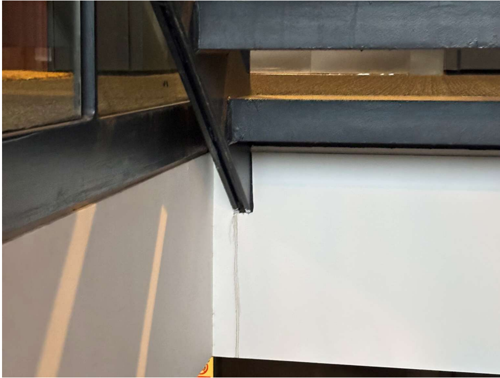
Figure 26 – Minor staining to the plasterboard from run-off from the steel staircase.
