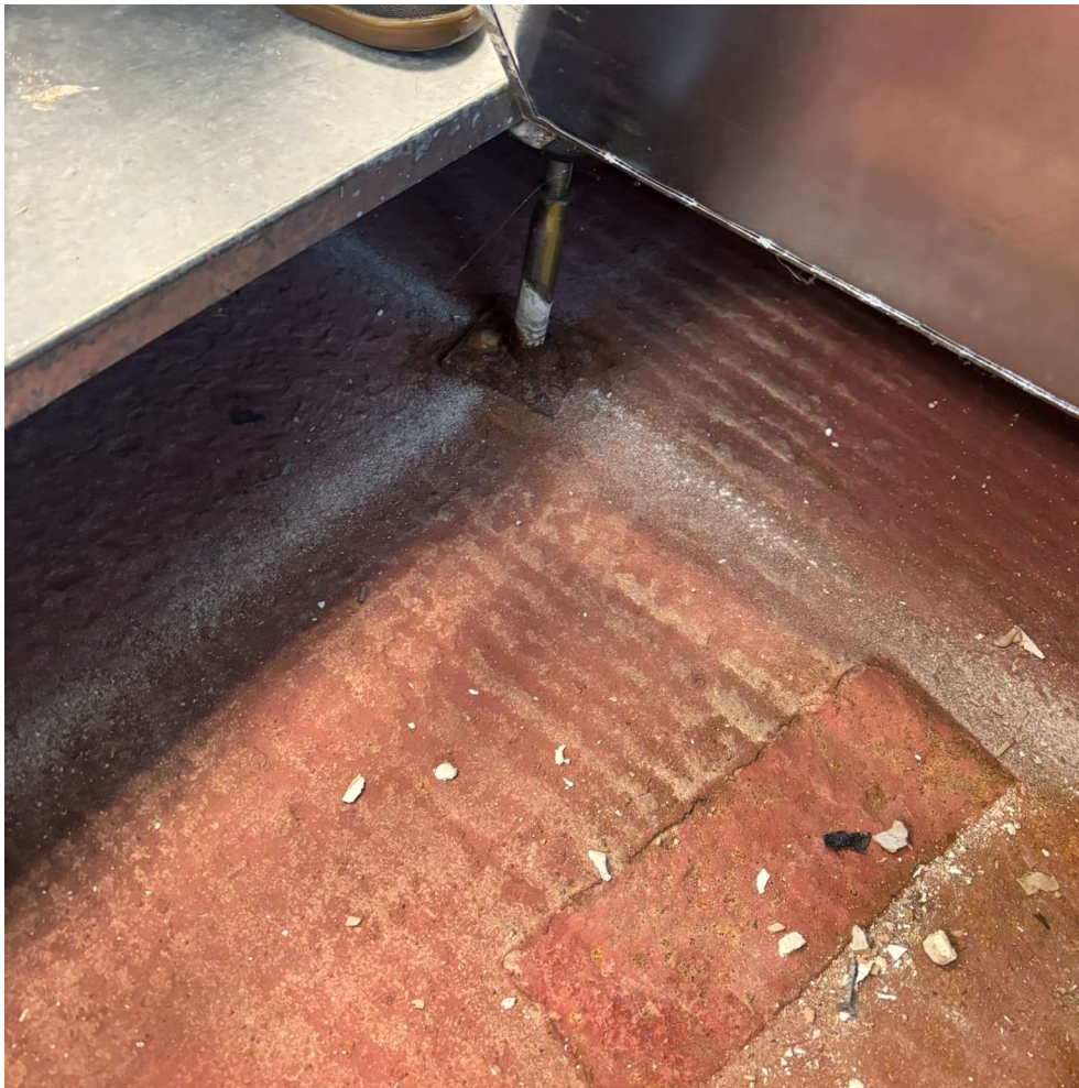
Figure 24 - Typical Photograph of corrosion to raised access floor support
