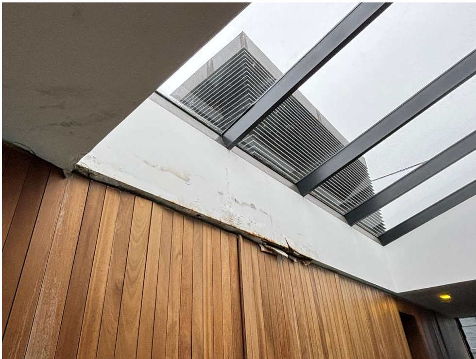
Figure 22 - Typical photograph showing evidence of water ingress, risk of corrosion to steelwork
