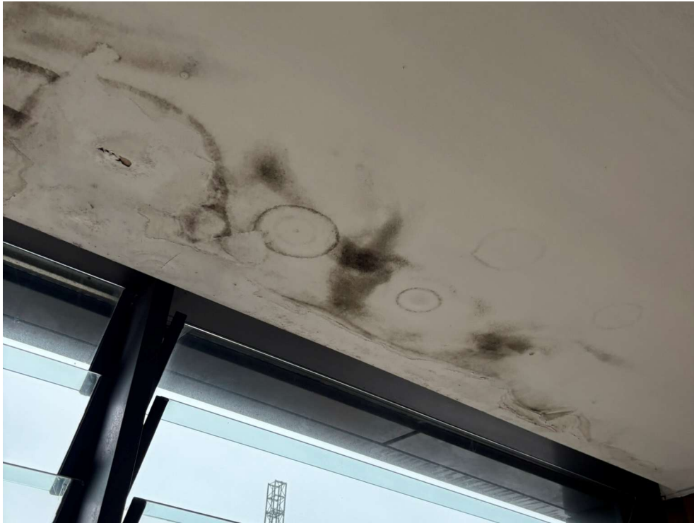
Photograph 1 - Typical Photograph of Water Ingress
