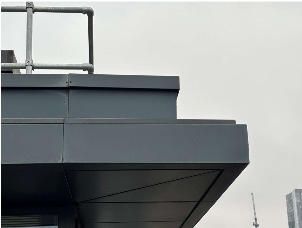
Photograph 20 – Deflection to Roof Gridline 15
