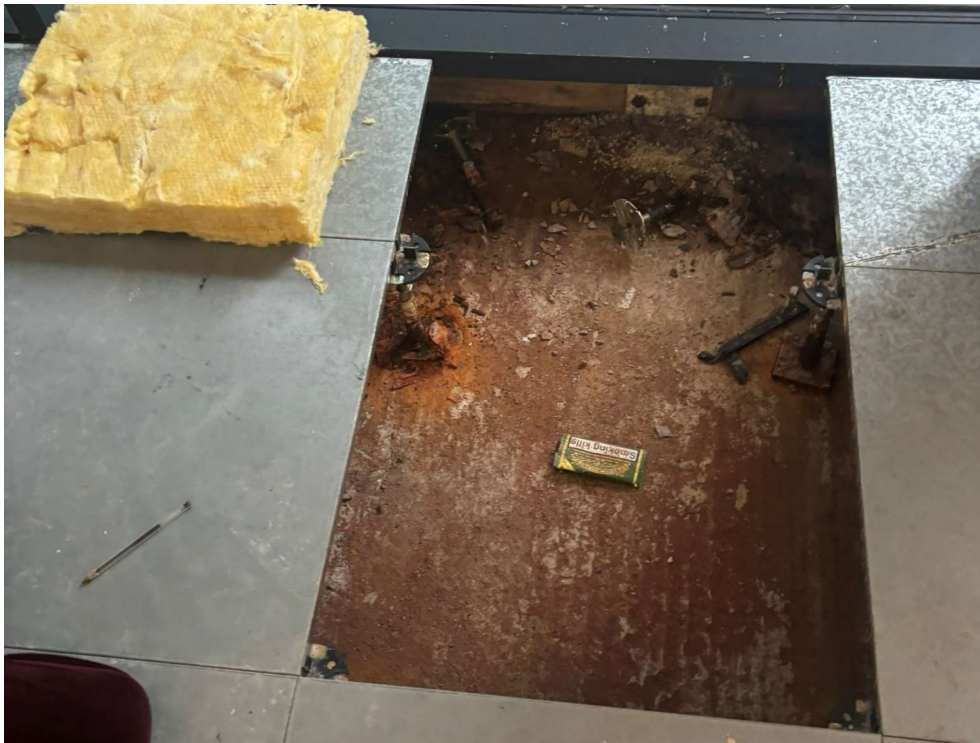
Photograph 7 - Water Ingress Within The Ground Floor
