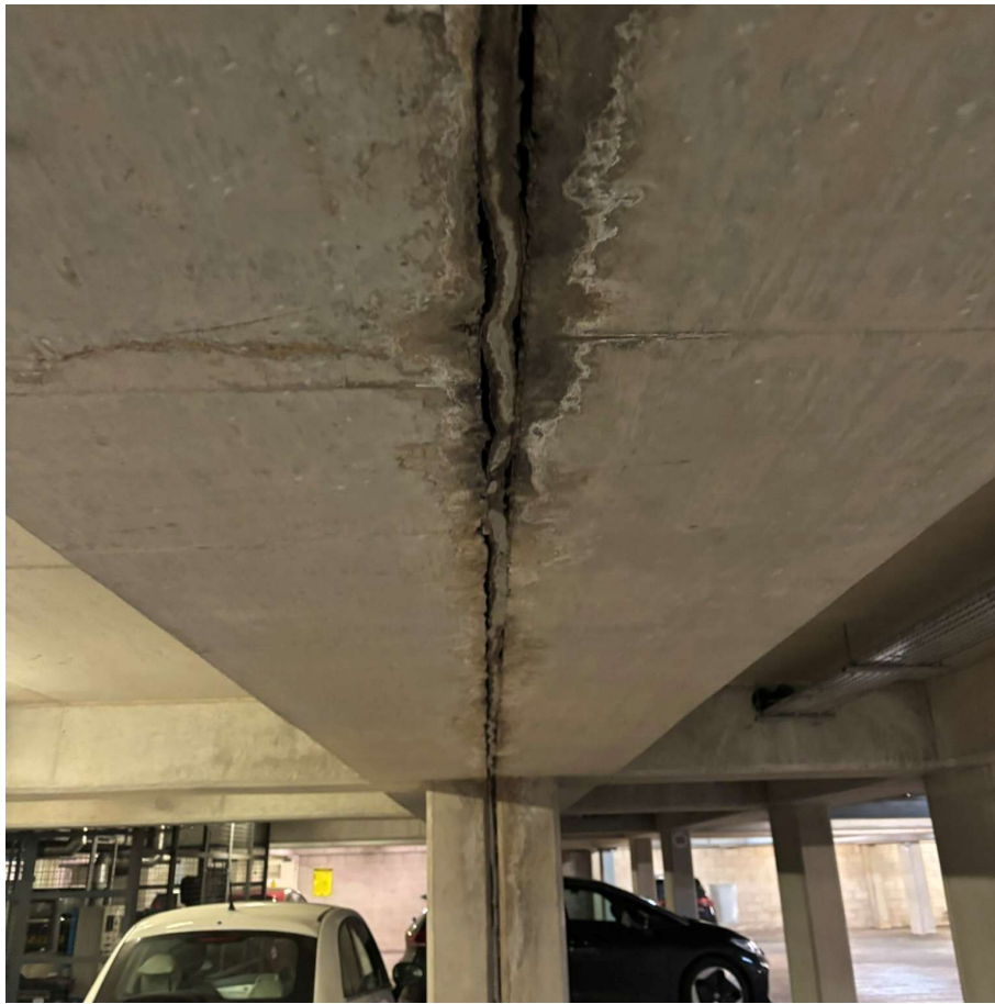
Figure 30 - Typical Photograph of Failed Movement Joint Plus Water Ingress
