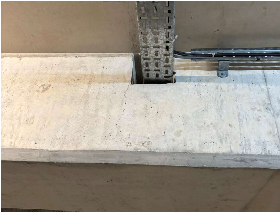
Figure 29 - Typical Photograph of Cracking Local to Service Opening in Basement Beams
