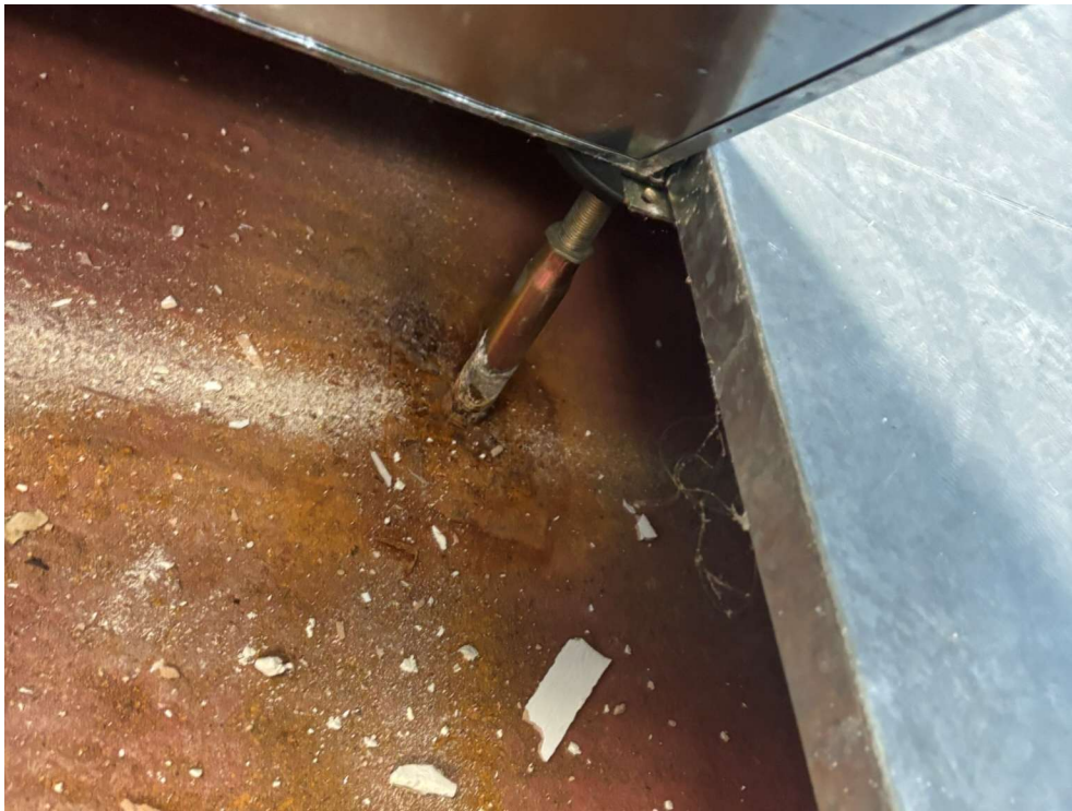
Photograph 9 - Corrosion To The Raised Access Floor Leg Supports
