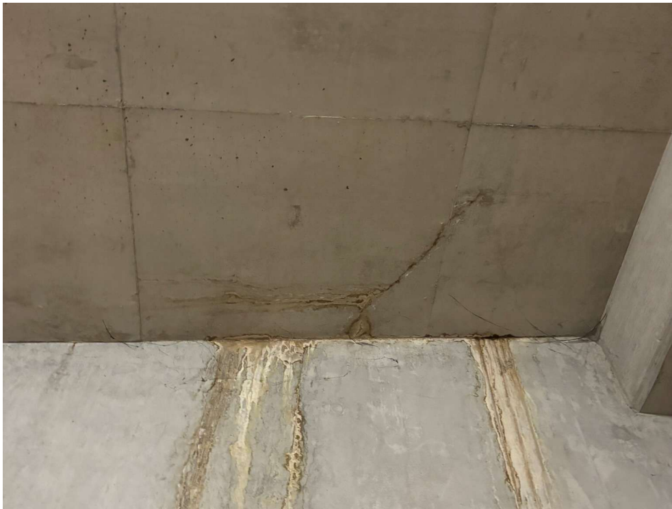
Photograph 17 - Hairline Shrinkage Cracking To Soffit Of In-Situ Reinforced Concrete Basement Floor Plate
