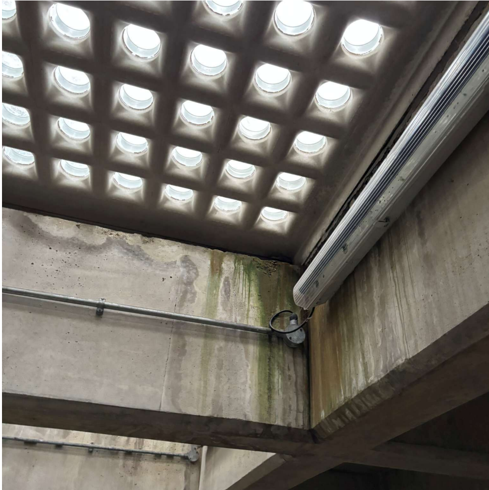
Figure 27 - Typical photograph of water ingress at joints of basement lightwell
