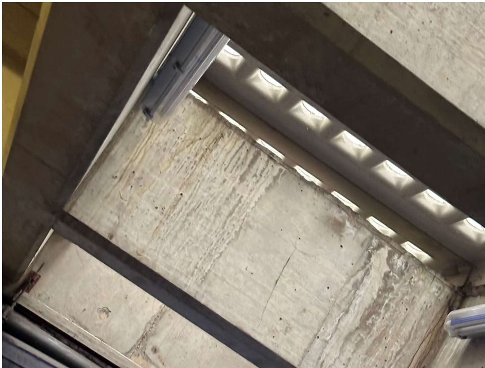
Photograph 13 - Water Ingress Within Basement Areas External to the Main Building Footprint at the Transition Between In-Situ Deck and Natural Light Floor Construction.
